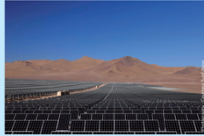
Project: CAP (Amanecer Solar) Megawatts: 101.2 Location: Copiapo, Chile
